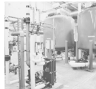
Big water filter system
