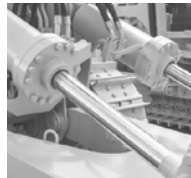
Hydraulic doors and split
